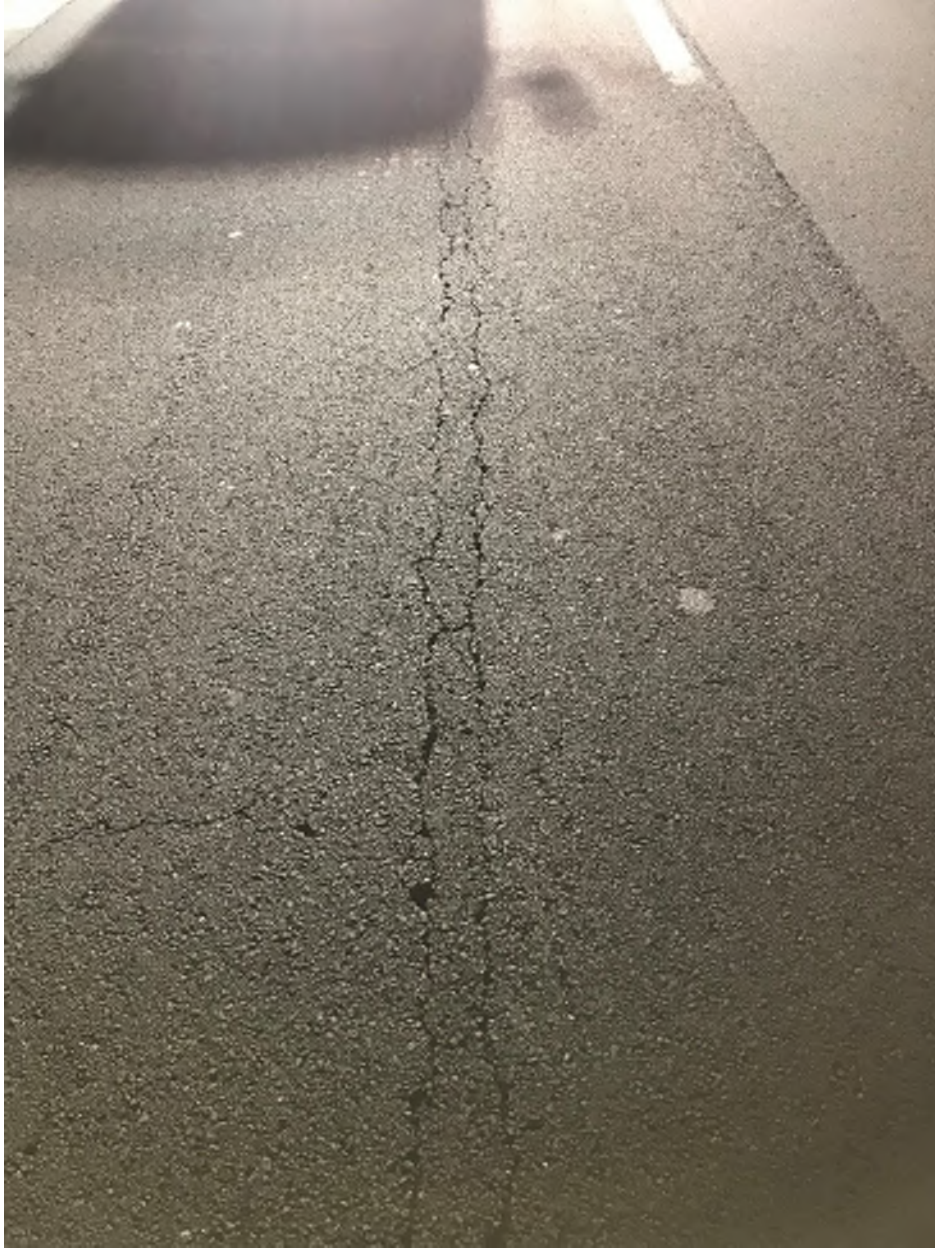
Photo 5 – Typical Longitudinal Cracking noted as Alligator Cracking due to appearance and location in wheel path. Likely caused by underlying longitudinal joint
