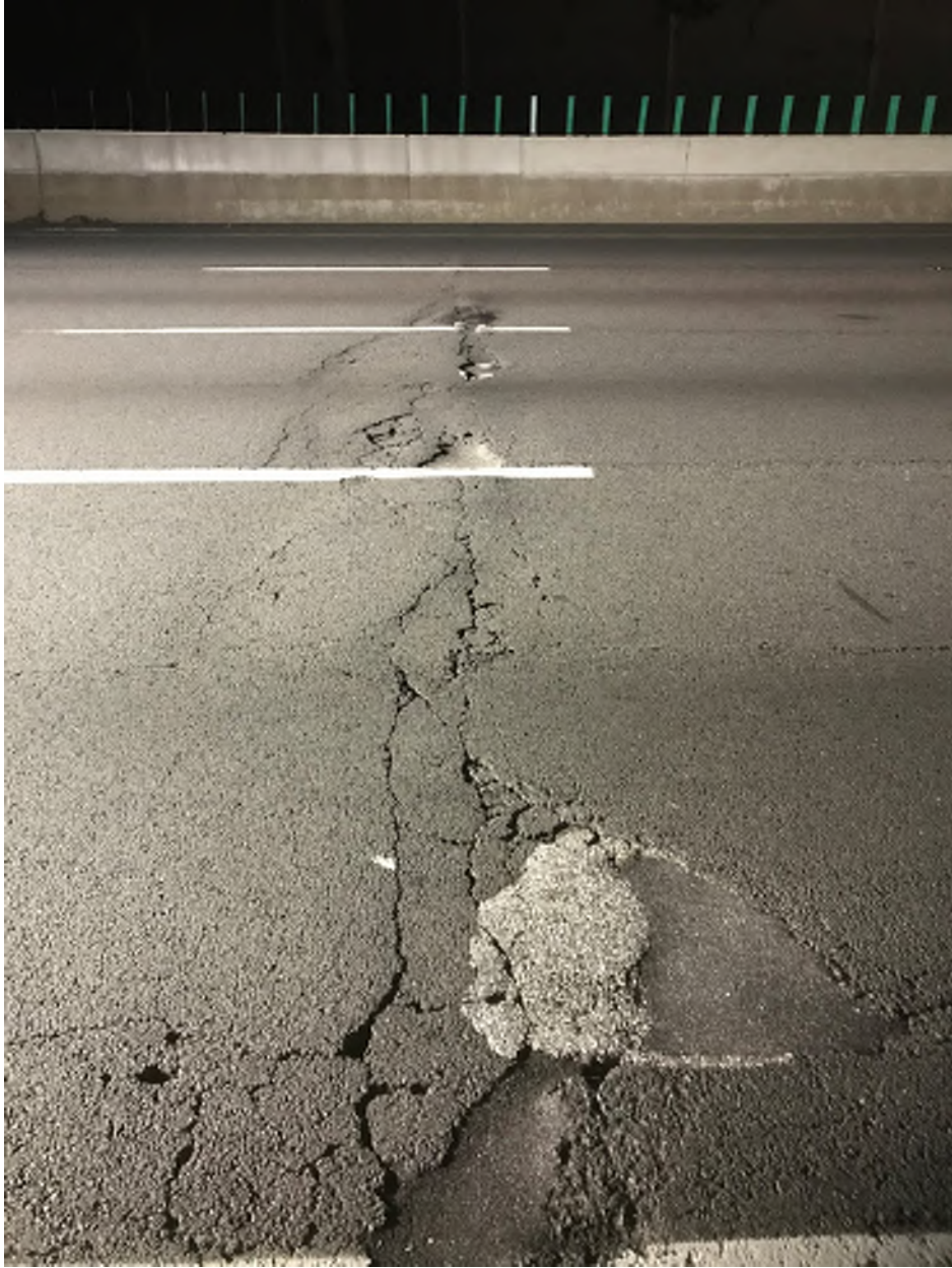
Photo 4 – Typical Type 3 Joint/Crack (Note presence of patching)
