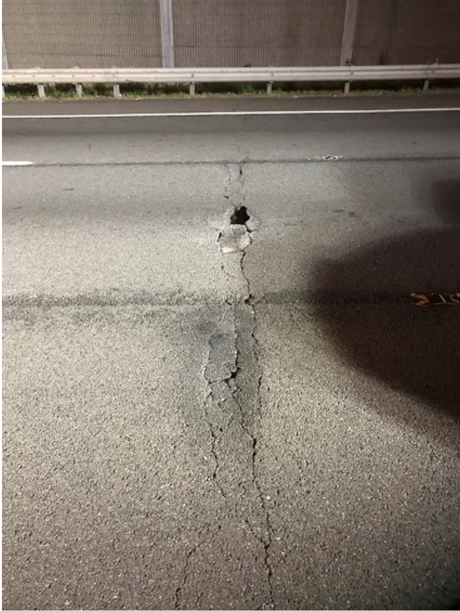
Photo 3 – Typical Type 3 Joint/Crack
