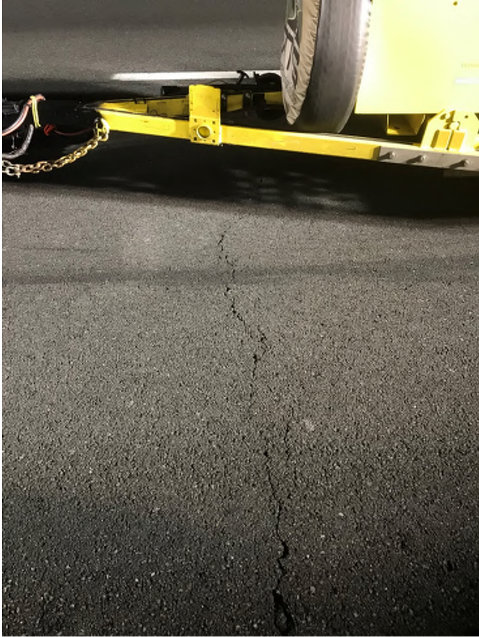
Photo 1 – Typical Type 1 Joint/Crack
